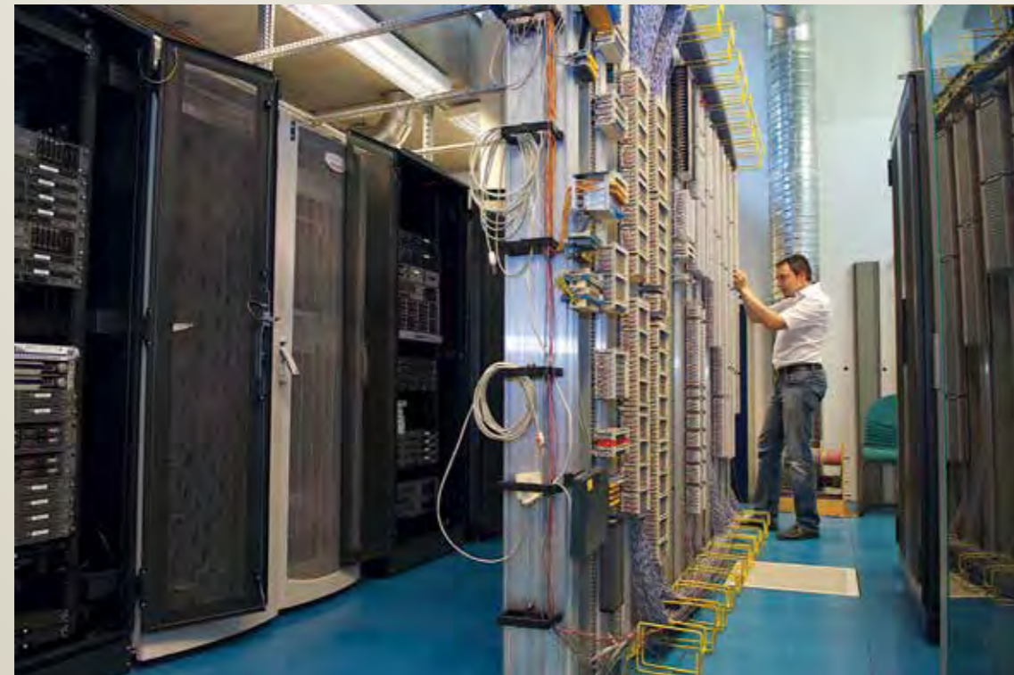
The Court's server room – the core of the IT system.
